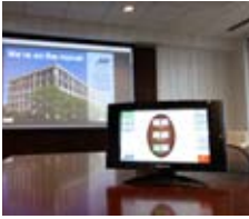
Crestron room control
